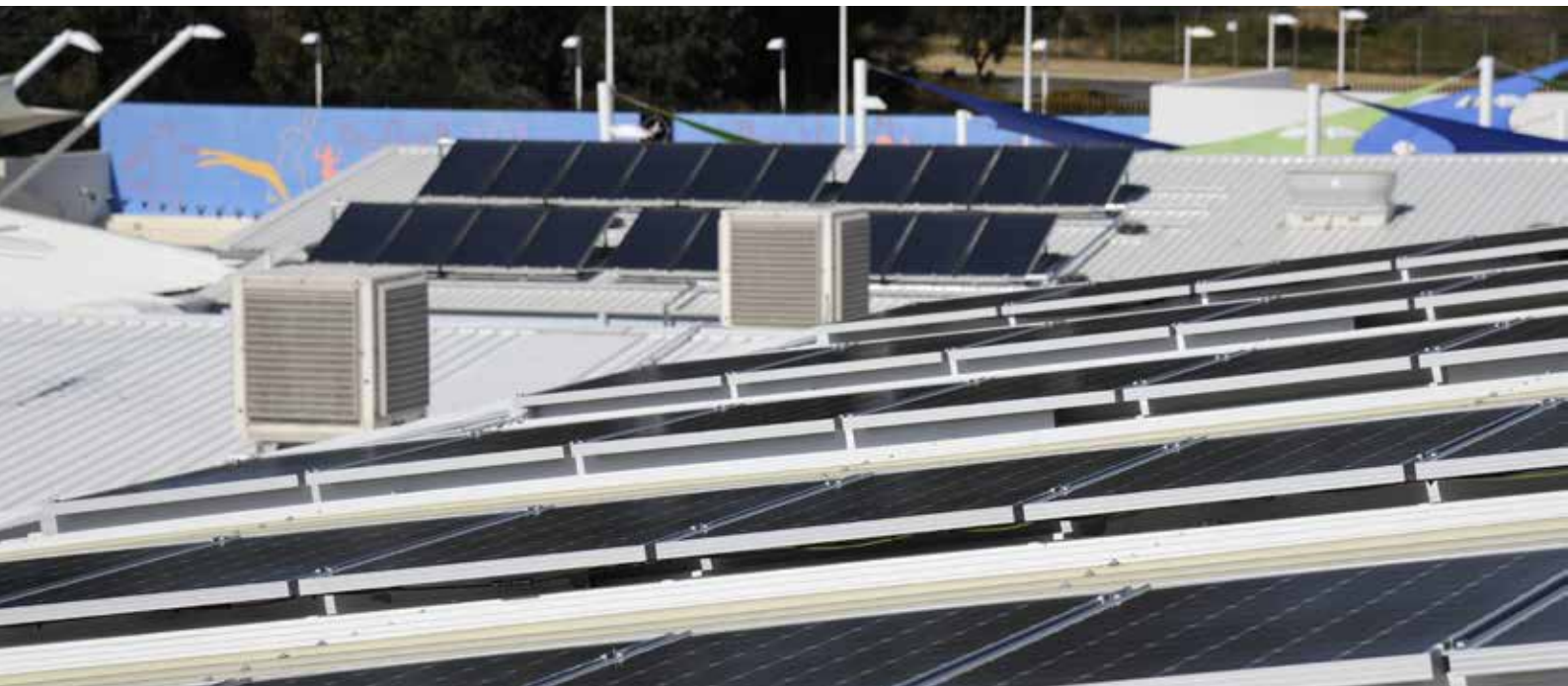
Photovoltaic cells on the roof of the Craigie Leisure Centre
