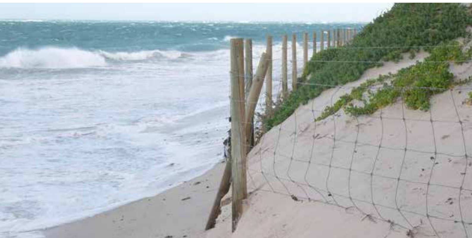
Coastal erosion along the City of Joondalup coastline
