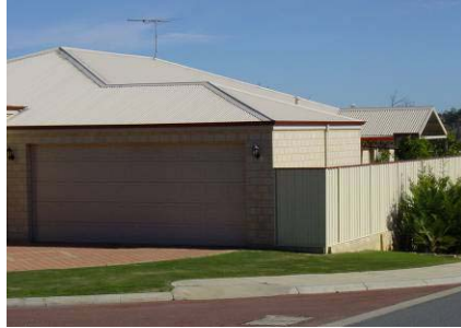
Photo 1: Unacceptable corner treatment
