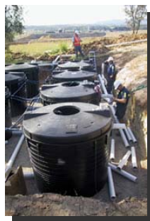
Ashton mine sewerage treatment plant, Hunter Valley, NSW
