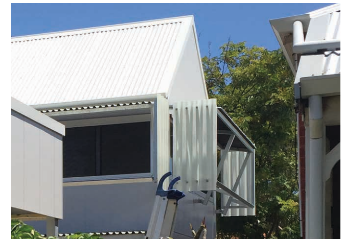
Photo G3.10c This window hood effectively restricts overlooking of the neighbouring property's rear garden without compromising amenity for the dwelling
