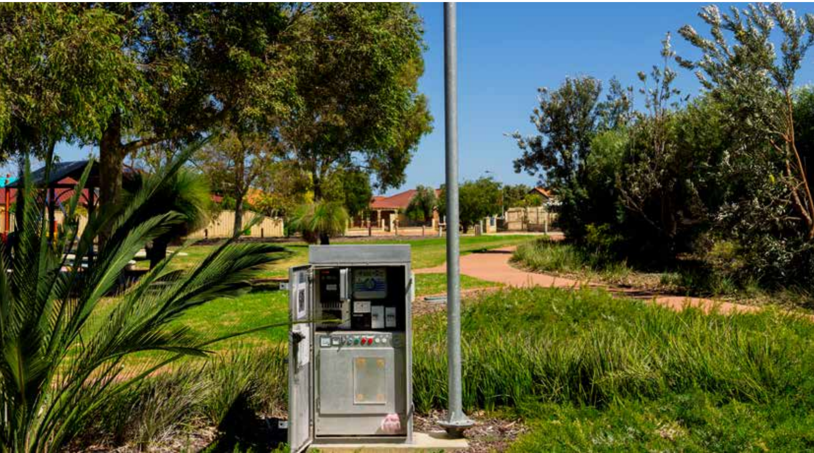
Irrigation controller at Santa Ana Park (Currambine)
