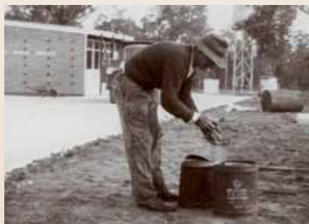
Tom Ostle cleaning his hands after laying bitumen at the new Wanneroo Road Board office ca. 1960.
