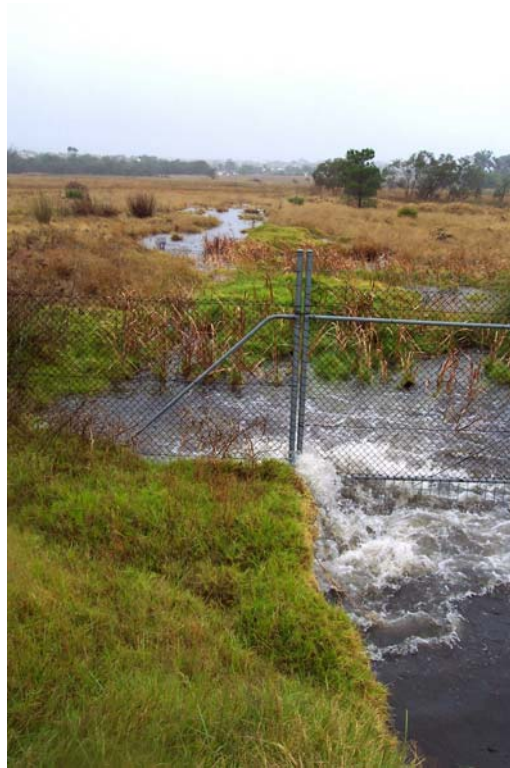
Figure 12a. In times of high flow rates after heavy rainfall, the untreated water from the Wangara Industrial area overflows directly into Walluburnup Swamp (Photos by John Chester taken in May, 2004).
