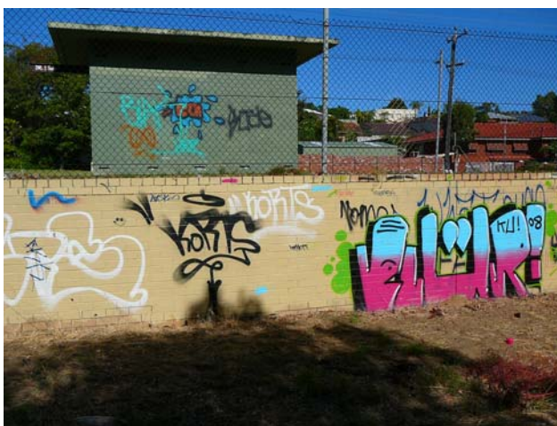
Figure 30. Graffiti at Lake Goollelal. Graffiti in the Park is an on-going problem and costs thousands of dollars each year to remove (Photo by Gary Tate).
