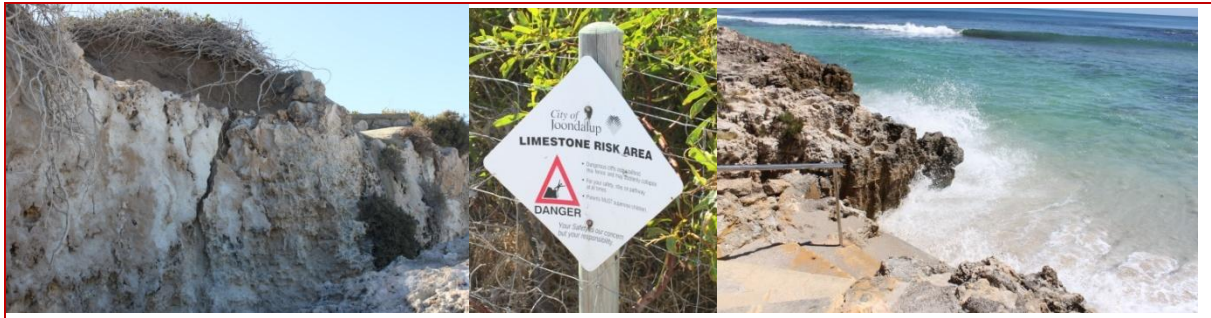
Figure 44: Limestone Cliff Risks and Management Issues
