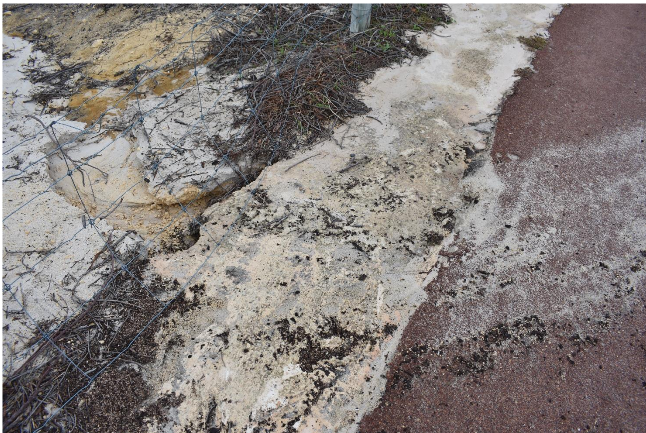
Figure 6: Runoff causing erosion off the dual use path into the adjacent dune swale
