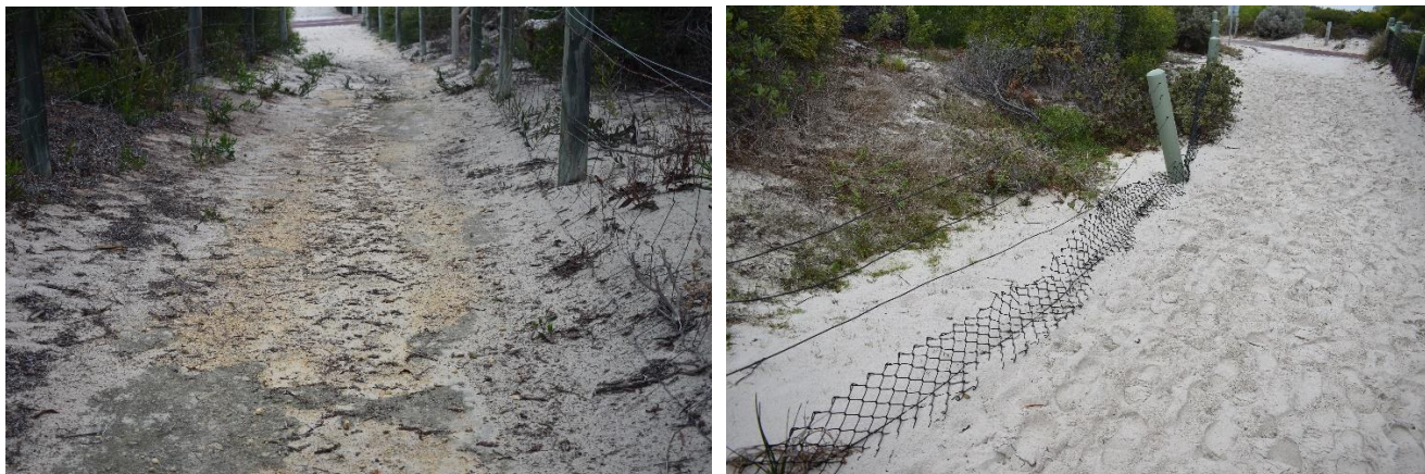
Figure 23: Pathway requiring maintenance (left), and subject to erosion (right)
