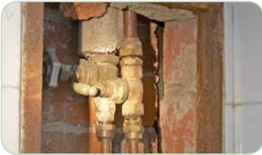
Friable asbestos lagging on pipes
