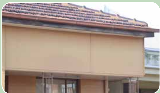
Asbestos cement sheeting in eaves
