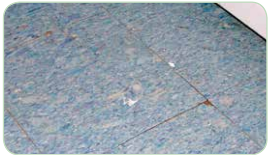
Typical old vinyl floor tiles that might have asbestos in the backing material
