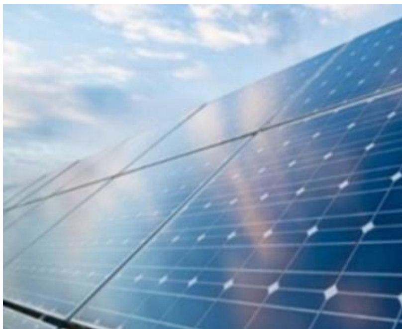
Figure 5-1 Rooftop PV system
